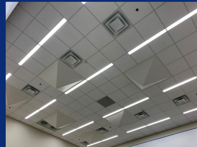
Acoustical Ceiling Diffusers in Area K
